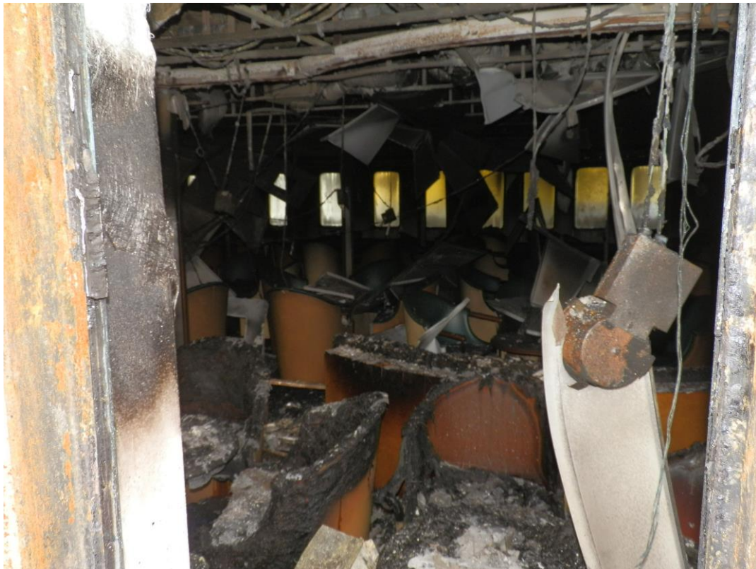
Figure 8: Capture of the port side accommodation lounge (deck 7)
