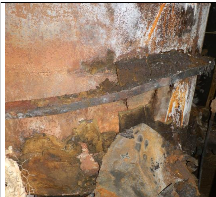
Figure 19: Part of the exhaust pipe inside the port funnel duct. The damaged insulation is visible in the lower part of the picture.
