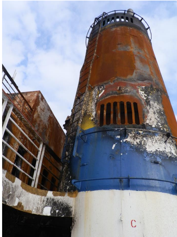
Figure 4: Capture of the aft side of the port side funnel duct with evident results of the fire
