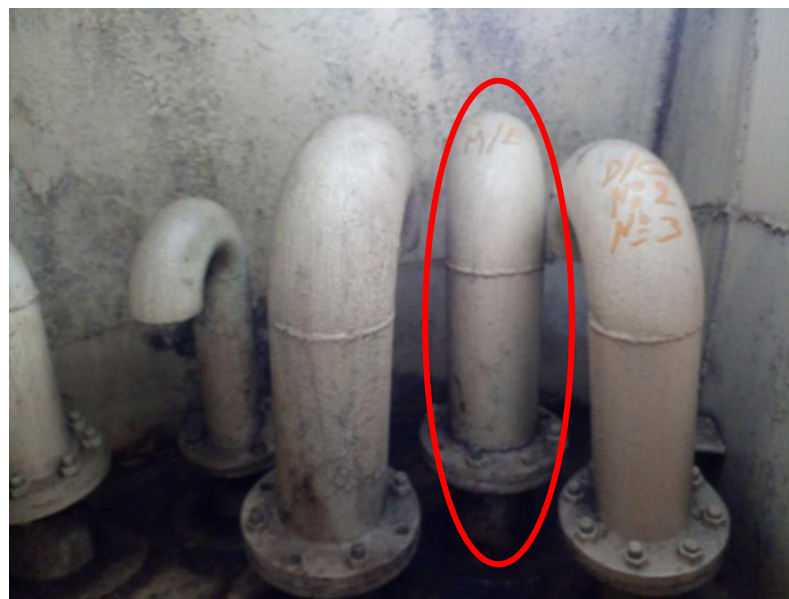
Figure 16: The air extractor pipe's ending (indicated) over the panel within the port funnel duct (photo captured after the repairs)
