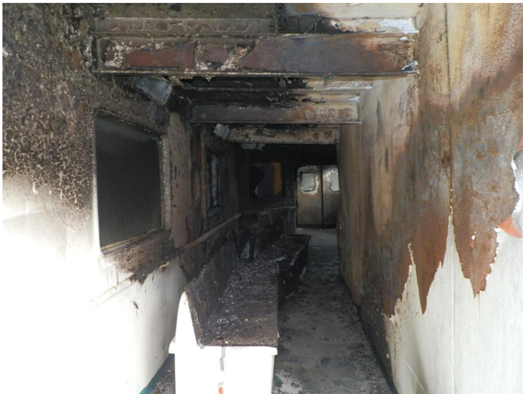
Figure 6: Capture from the external accommodation spaces at the port side of the vessel (deck 8)
