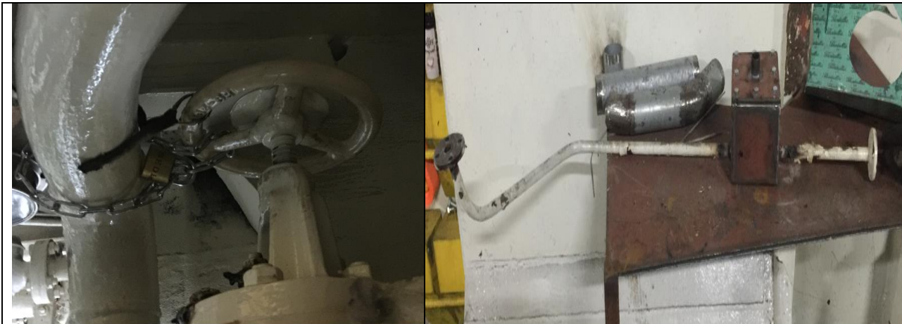
Figure 20: Left :The return valve secured with a chain and lock. Right: The alarm monitoring device ready to be fitted at the air extractor pipe of the return chamber.
