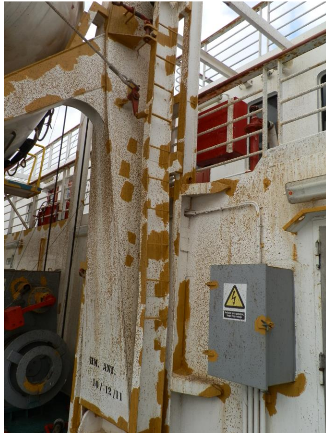
Figure 11: the area around the port funnel. Traces of the oily mixture spray are quite evident on the bulkheads (deck 7, port side)
