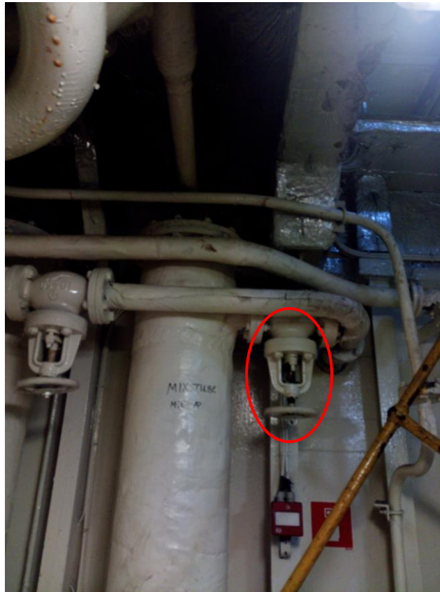
Figure 14: the valve from the Return Chamber to the fuel supply pipe, which was found damaged (photo captured after ship's repairs)
