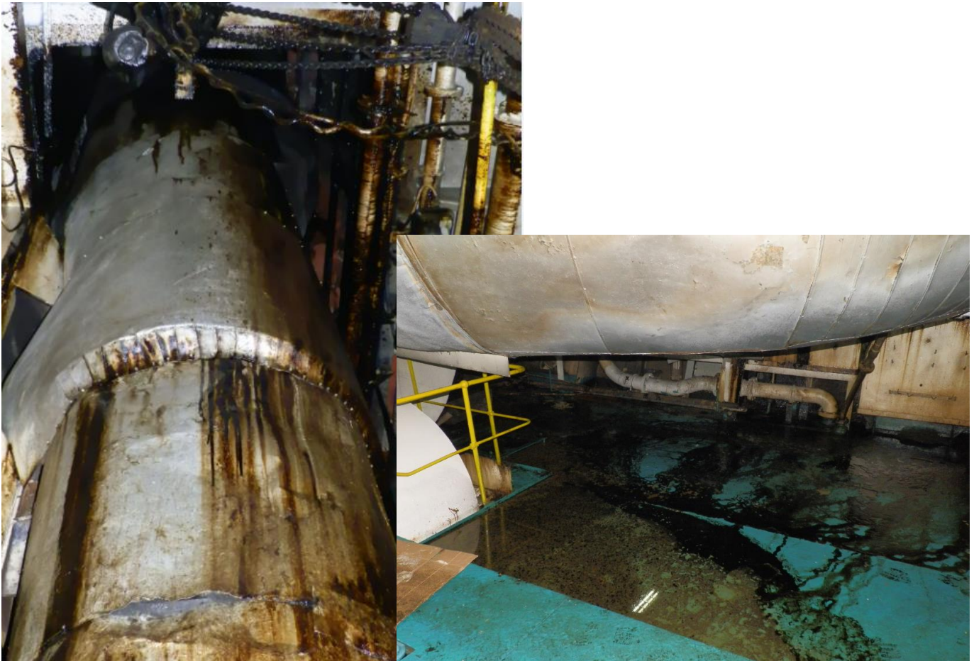
Figure 13: visible oil traces on the surface of the exhaust pipe and the port side main engine room
