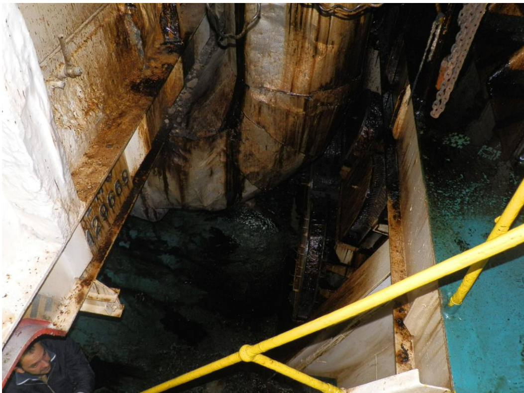
Figure 10: Capture of the floor of the engine room, right below the port funnel, with evident residues from the extinguishing process
