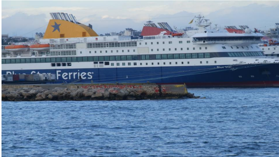
Figure 26. The damaged head of the breakwater. View from outer port section.
