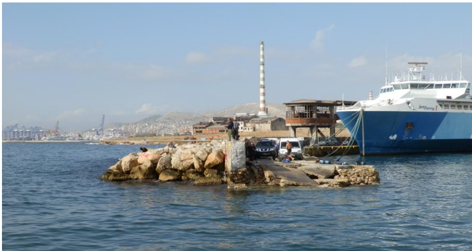
Figure 24. The damaged head of the breakwater. Abeam view.
