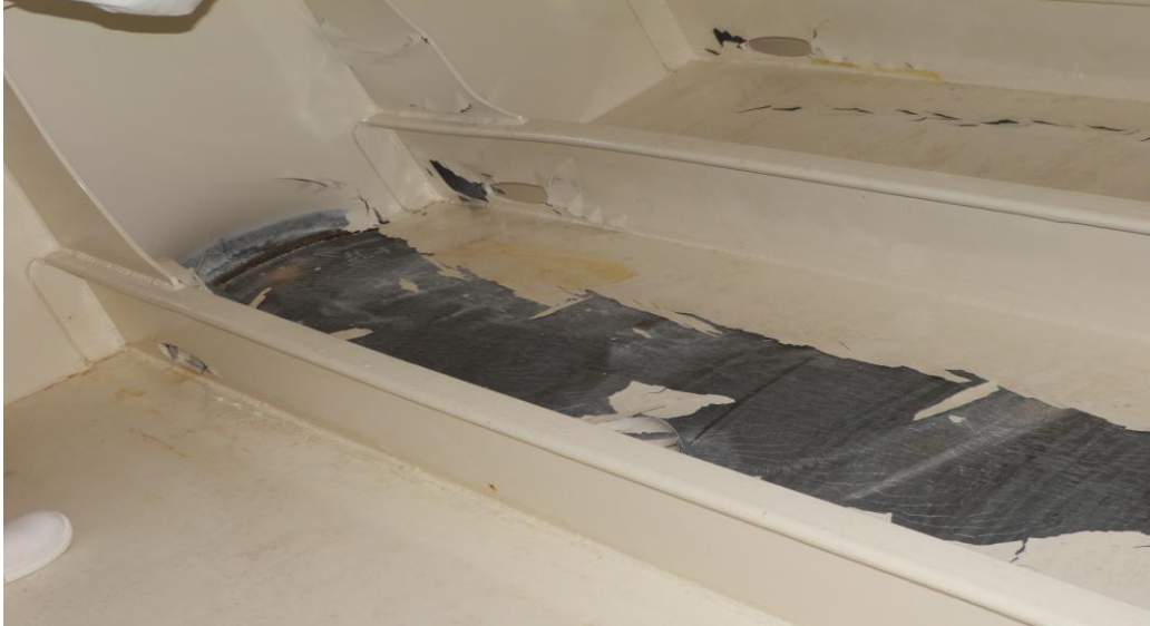
Figure 31. The deformations sustained on the hull plating under the waterline caused by the contact on the breakwater substructure.
