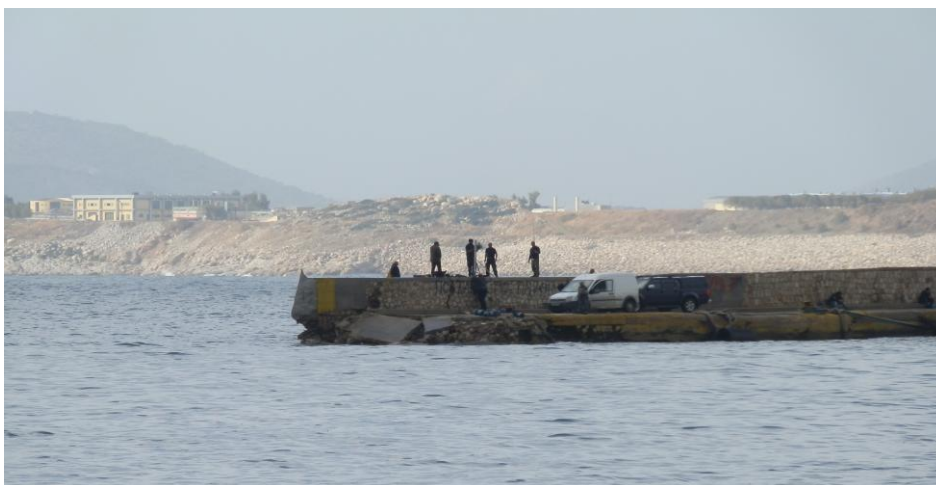
Figure 25. The damaged head of the breakwater. View from Prolimenas section.
