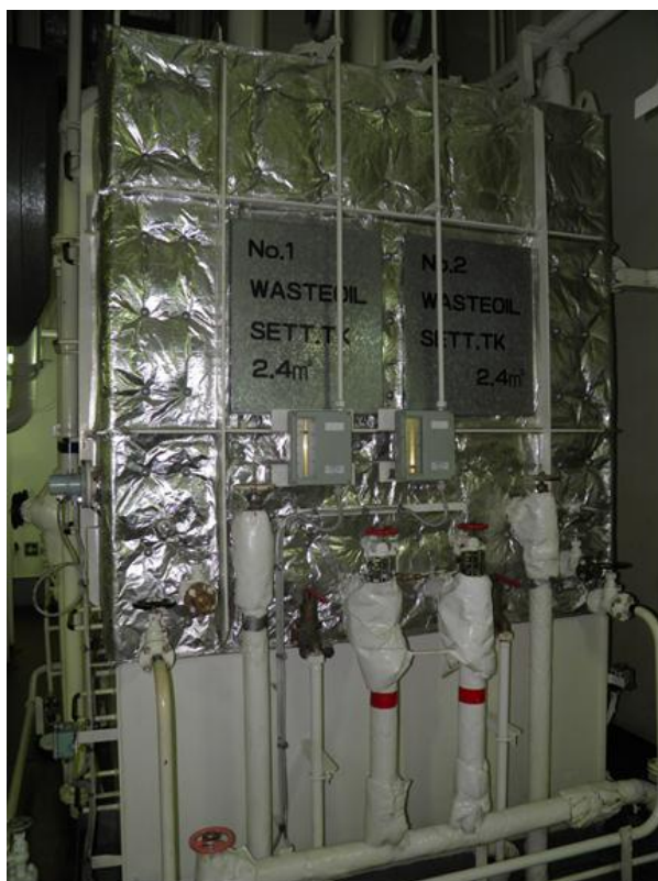
The Waste Oil Settling Tanks
