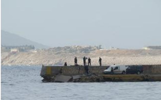
Figure 2: The damaged head of the breakwater.
