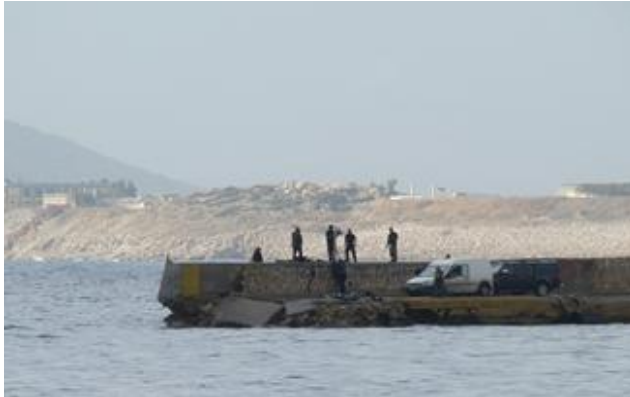
Figure 2: The damaged head of the breakwater.
