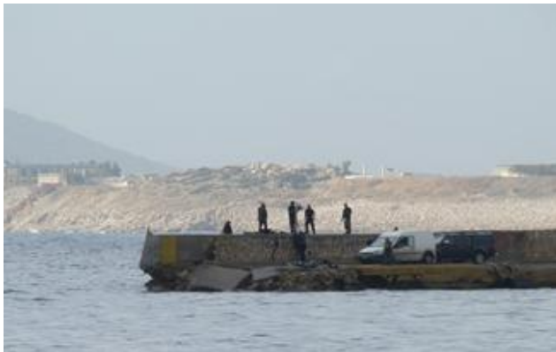
Figure 2: The damaged head of the breakwater.
