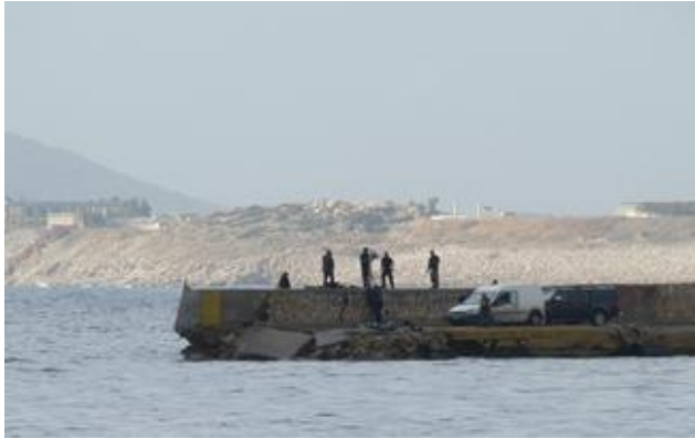
Figure 2: The damaged head of the breakwater.
