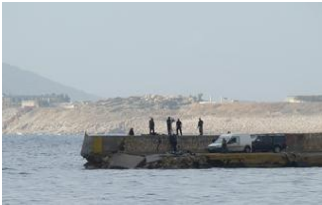
Figure 2: The damaged head of the breakwater .
