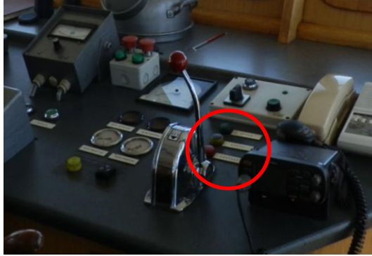
Picture 4: View of the direction drive control lever where the indicative position lights are shown (inside the red circle)
