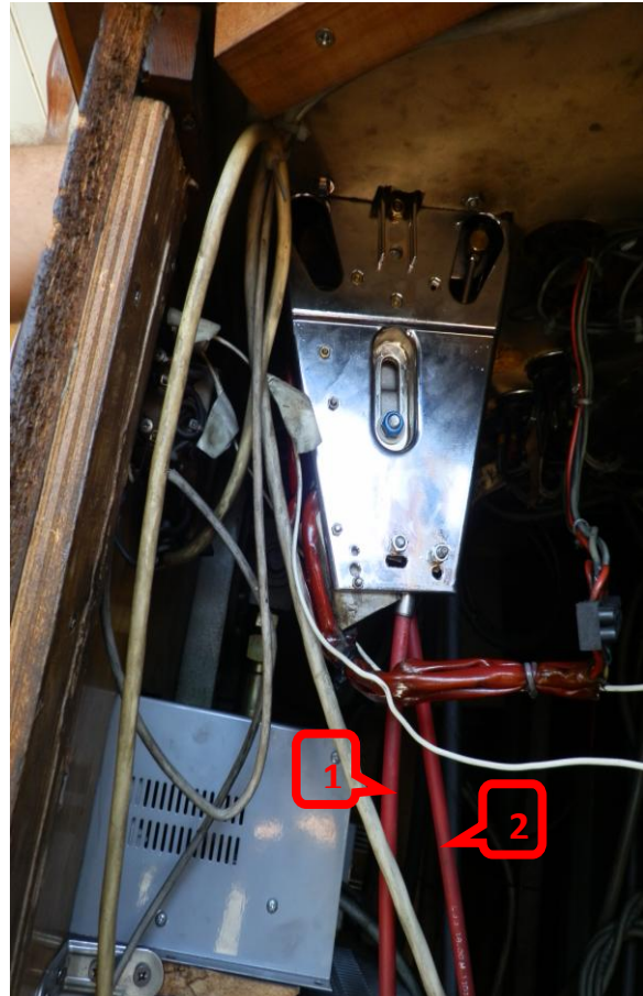
Picture 5: View of the lower part of the control system where the cables towards the engine room have been marked.
