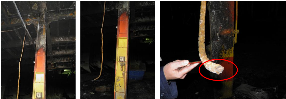
The aft side of the pillar, between frames 219-221, and the cut cable.
