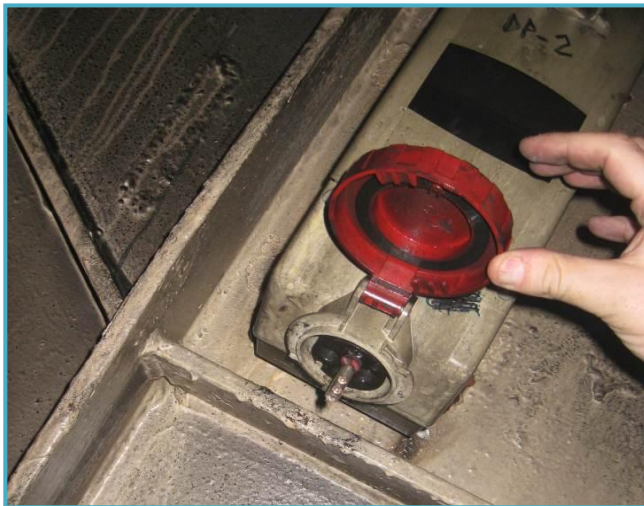
The cable extension (extension cord), that was connected to a refrigerator truck and which is rated as one of the possible fire ignition points. The damaged side of the cable that ended at the refrigerated truck is shown and the plug which was connected to the socket DP2.
